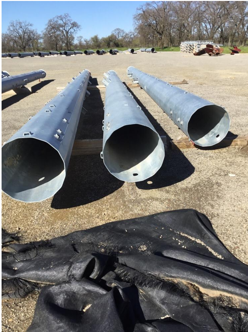
Photo 3: Staged materials at LZ 4/31. The CPUC EM verified that crews were reminded to check inside staged materials for nesting birds prior to moving.
