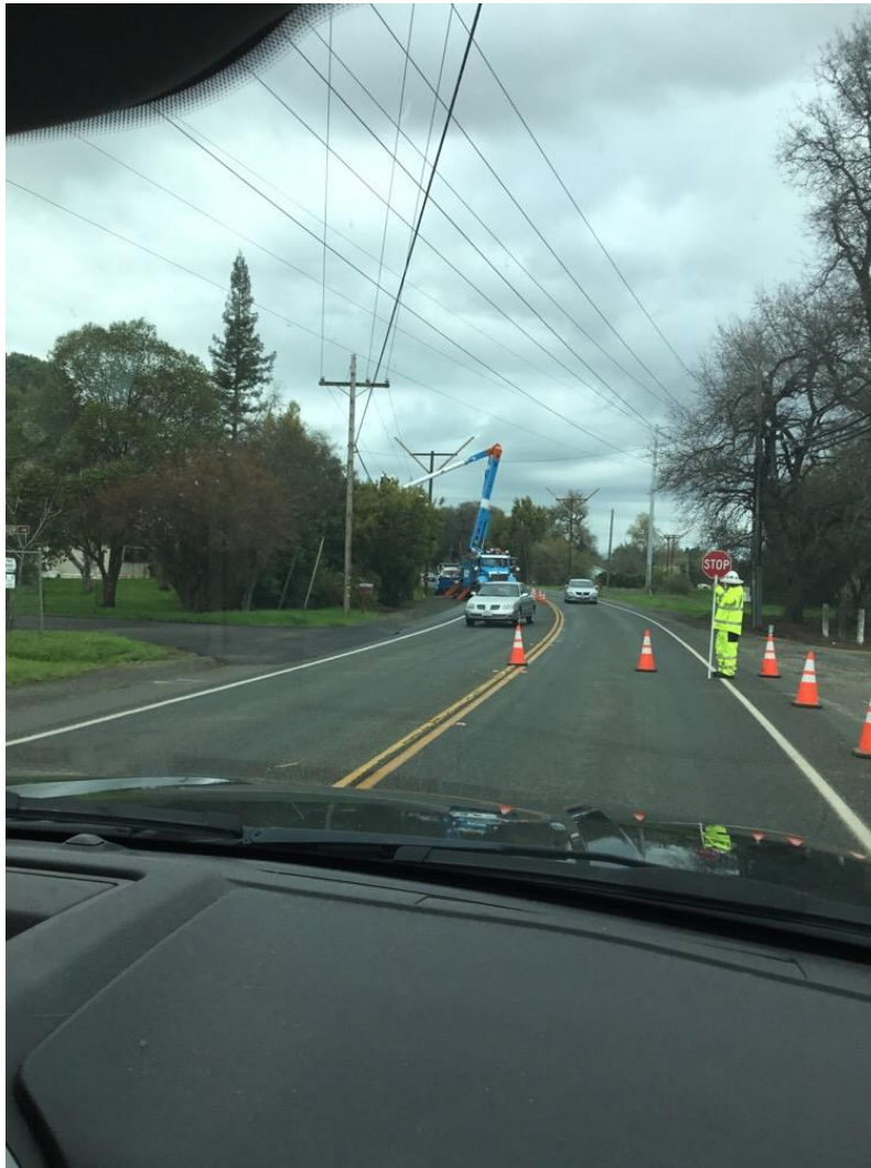
Photo 5: Temporary traffic controls were observed during construction work along Lincoln Boulevard in compliance with APM TRA-1.
