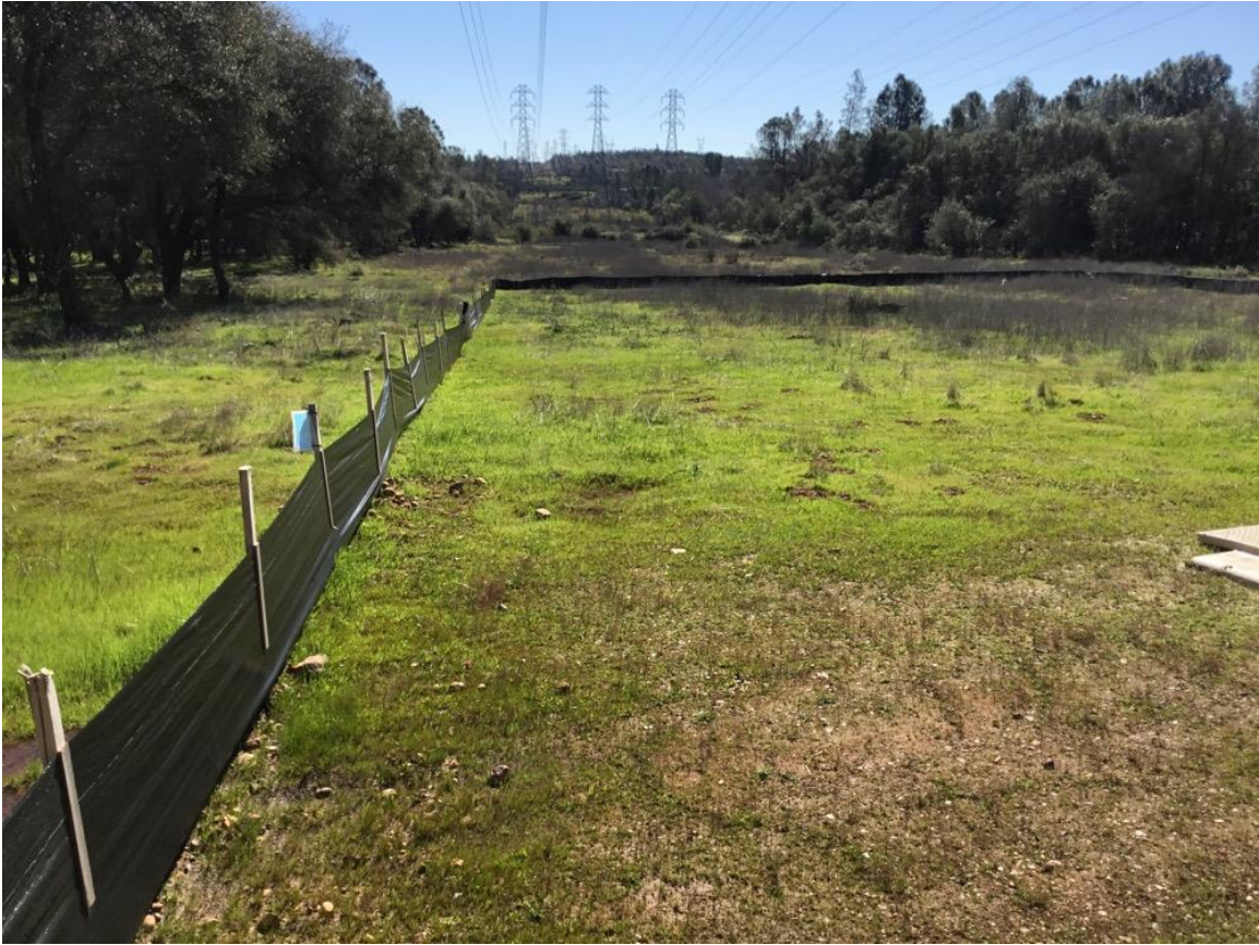
Photo 4: Installed silt fencing BMPs were observed to be in good condition near Landing Zone 1/11, in accordance with APM HYDRO-1.
